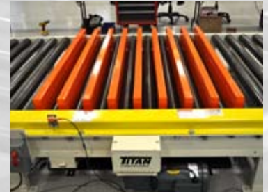
Pallet Lift in CDLR
